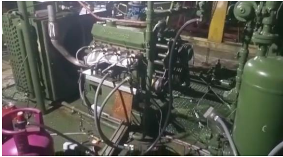
Figure 3. Gas Jack Compressor
